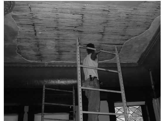
International Fine Art Conservation Studios is restoring the library ceiling after it collapsed in August.
